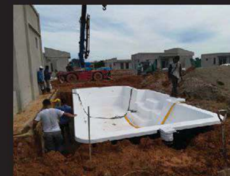
Total 53 units Hydro One Fiberpool (model MAURITIUS) supplied & installed at ECK Hijauan resort development project at Kulim, Kedah.
